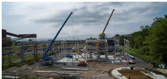
Cogeneration plant BE-TO Sisak
